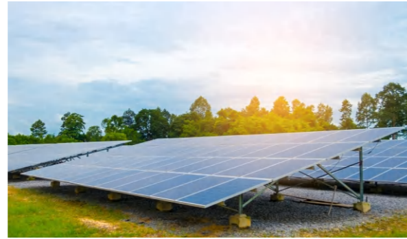
Ground Mount Racking
